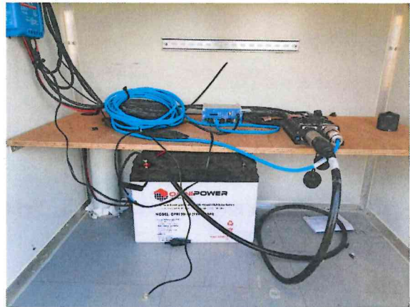
Figure 5: Inside the equipment housing
