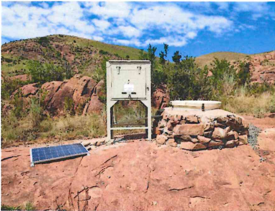
Figure 4: Complete seismic station
