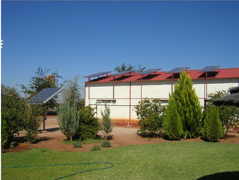
Large Solar Home System
