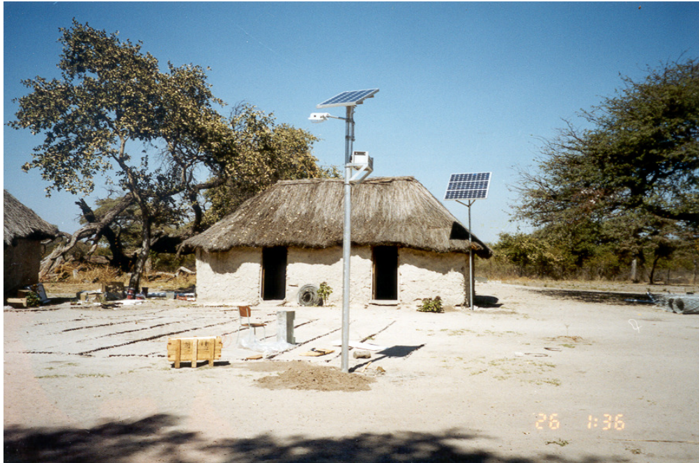
Medium Solar Home System with Street Light
