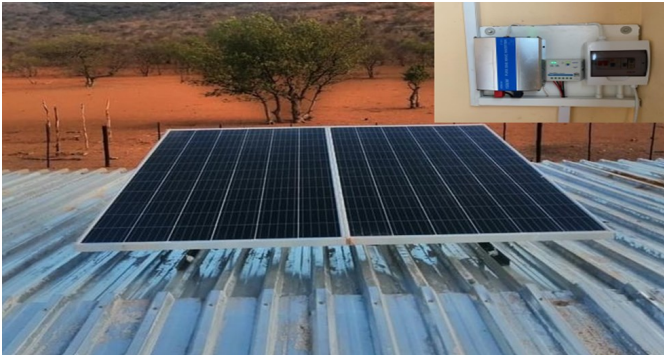
A Solar Home System typically has the capacity to power lights and devices such as radios, TVs, fridges and cell phone chargers. Energy Efficient Stoves for cooking and baking saves on wood, thus saving money and the environment.
