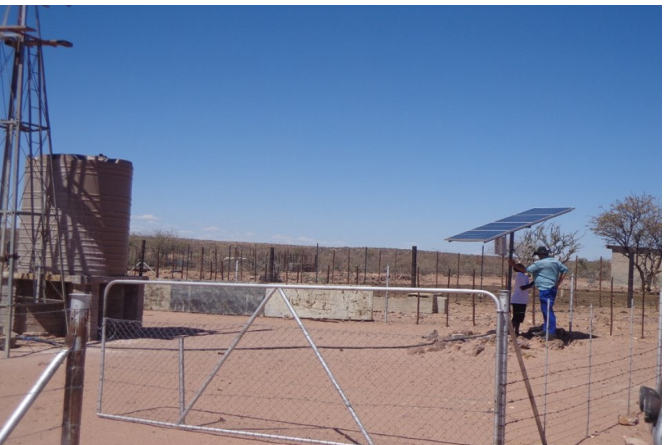
A Solar Water Pump uses water photo-voltaic panels to provide energy for pumping water for livestock and domestic use.
